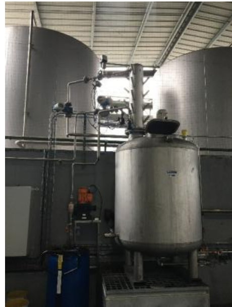
Automated concentrate dilution station
