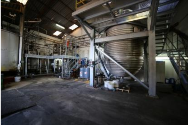
23 m 2 Dilution/manufacturing tank and dilution workshop
