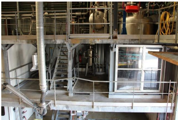
Stainless Steel filter drier: 3,000 litres (working pressure: vacuum/atmospheric pressure) Processing of 2,000 kg of plant materials per week.
